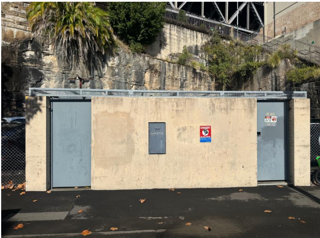
Figure 6: Existing Substation viewed from Hickson Road, facing east
